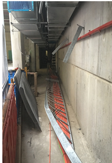
Photograph 2: Dropped cable tray
